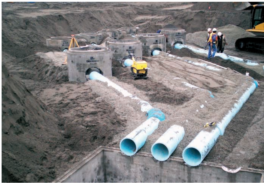
Deltaport installed 14 Stormceptor stormwater treatment systems, in addition to the original 43 such units installed during Stage 1 development in 1996.
