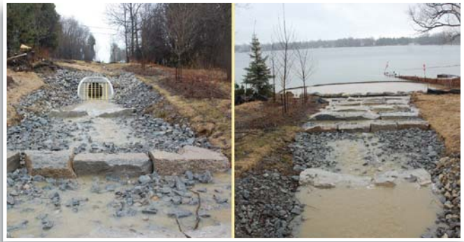
The runoff exiting from an underground stormwater treatment device should not contain this level of pollutants.
